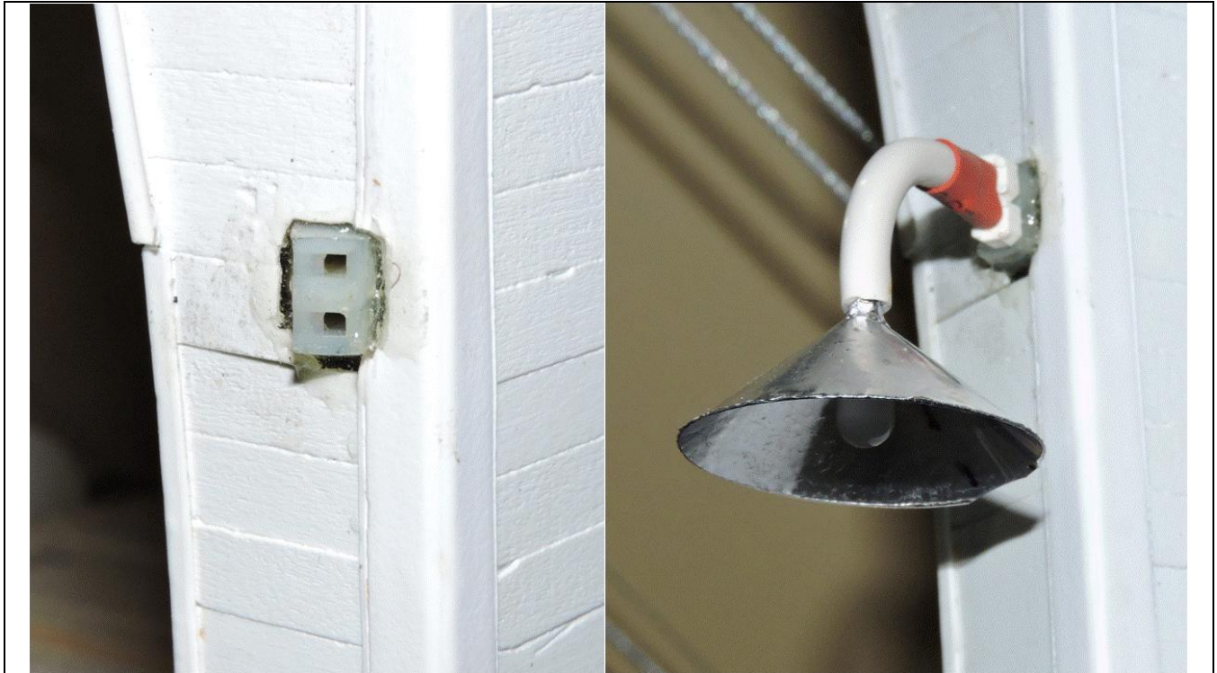
Figure 4. Tram Station Light Fixture Mount and Mounted Light
